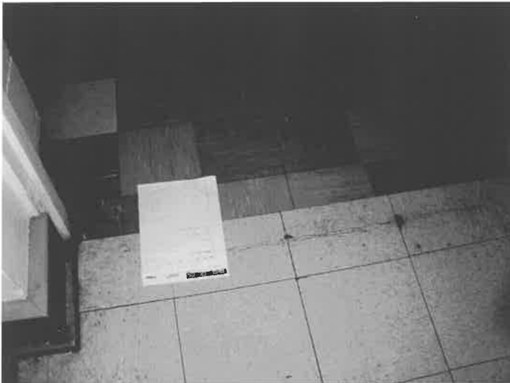
Photo No. 2. Photo of 9" x 9" floor tile and 12" x 12" floor tile typical throughout the main building.
