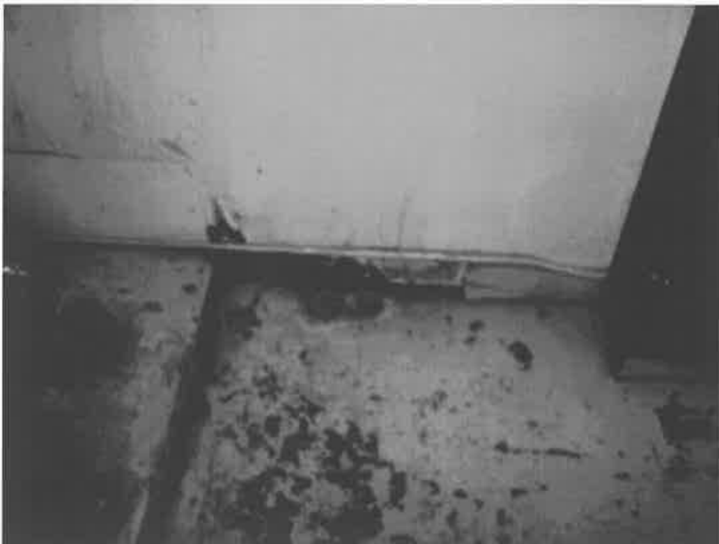
Photo No. 4. Photo of drywall typical throughout the building.
