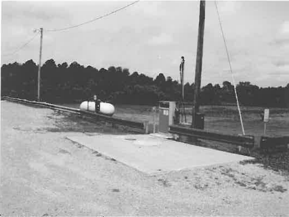
Photo No. 7. Looking northwest at gasoline fueling area consisting of a pump and underground storage tank.
