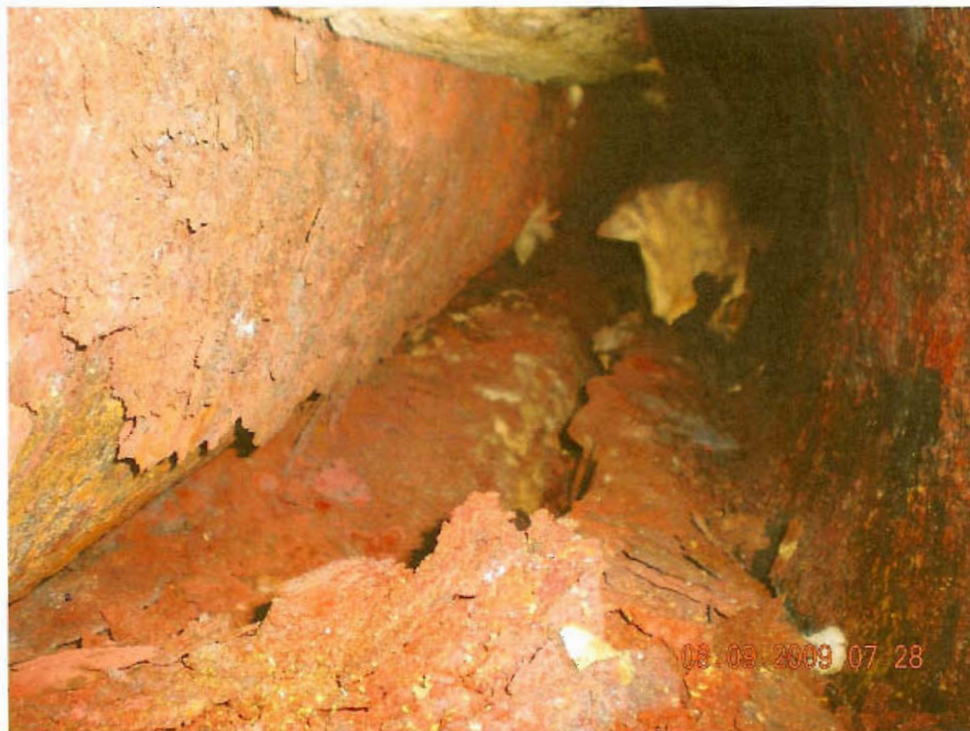
Corroded Steam Pipes
