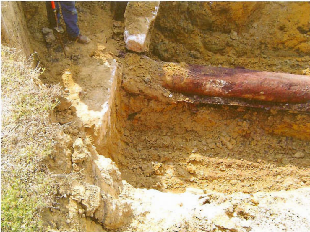
Corroded Steam Pipes
