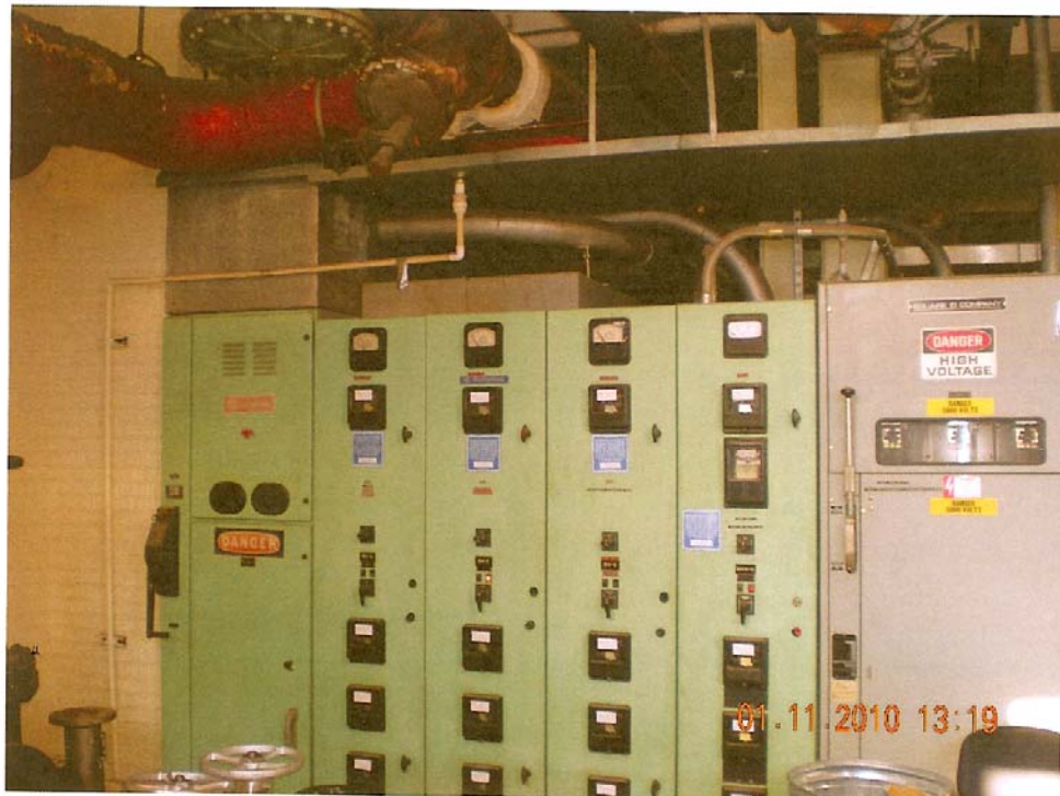
1929 Electrical Switch Gear
